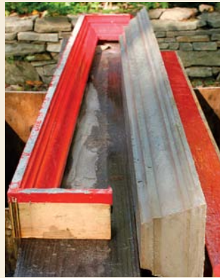
Taped for easy release. Lining the mantel form with housewrap tape makes dismantling the form easy. Blue masking tape works equally well.
